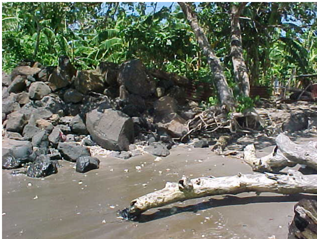
Erosion at the end of the village seawall at Sataoa.
