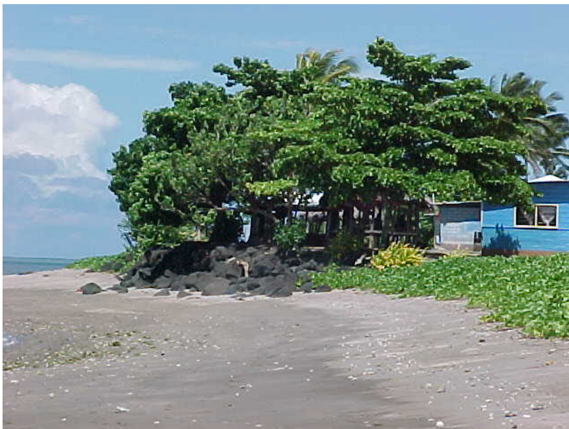
Village seawall in front of church house at Tafitoala showing degree of erosion around the end of the wall.
