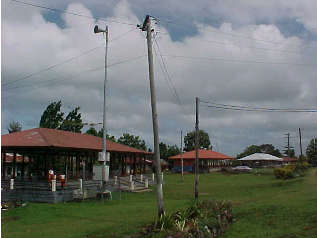
Telecommunication s Tower at Vaito'omuli on the seaward side of the road in the CFHZ. Equipment box raised above flood level.
