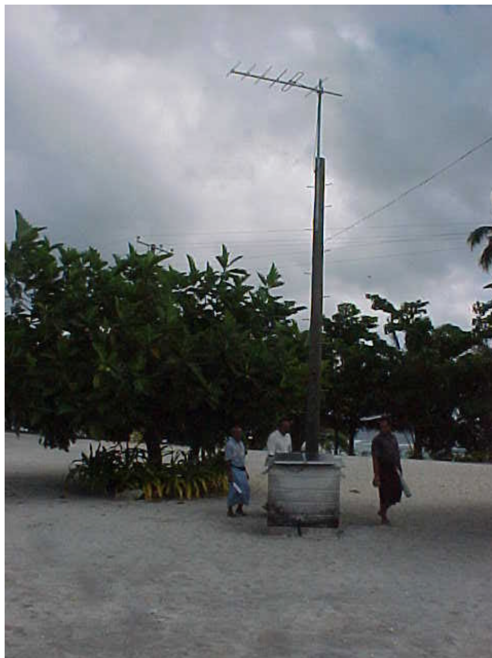
Microwave tower and equipment box located in the CEHZ and the CFHZ.
