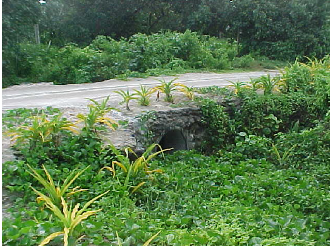
Drain under coastal access track showing sand formation spilling over the edge.
