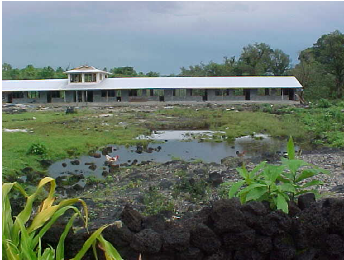
New primary school at Sale'aula built in CFHZ. Floor level raised but grounds still unfinished and subject to flooding.
