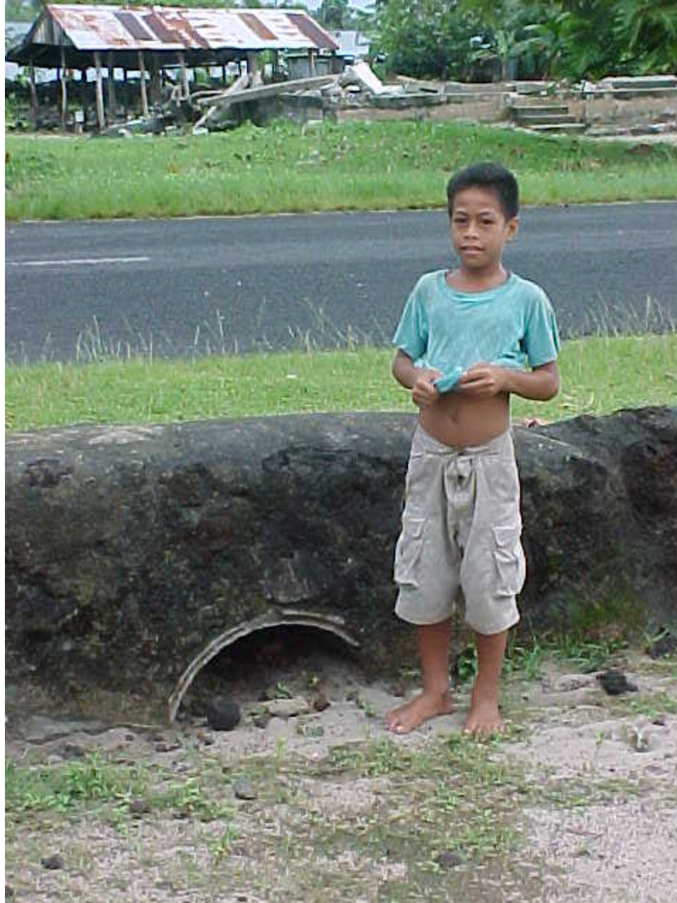
Blocked drain behind road at Sale'aula.
