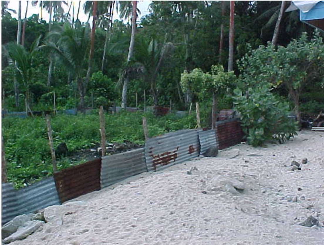
Wetland area used for gardens below the level of the house plot built up with sand. Old corrugated iron fence to retain the sand is ineffective and the plot and buildings are scouring out in heavy rain.
