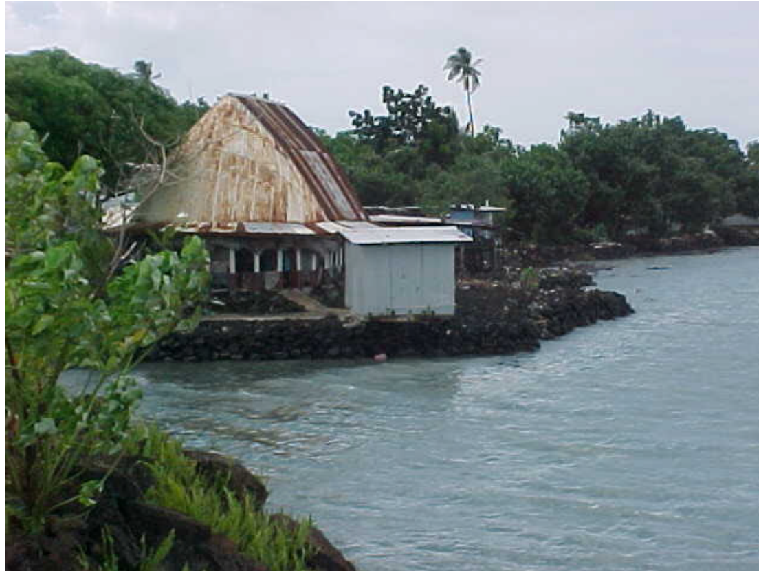
Reclamation at Foua close to sea level with toilets draining to the lagoon.
