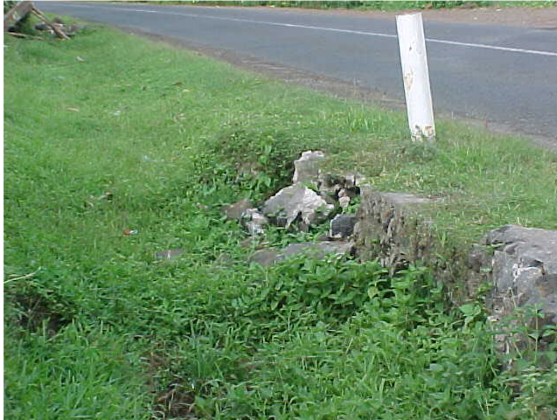
Blocked drain behind road at Saletagaloa.
