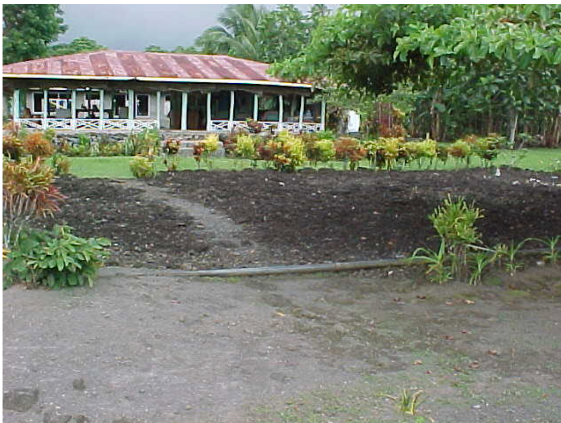
Flood area behind road at Vai'afai caused by culvert outlet invert being lower than surrounding ground levels. Exposed galvanised water pipe to be replaced by new PVC pipe under the EU Rural Water Supply Project.
