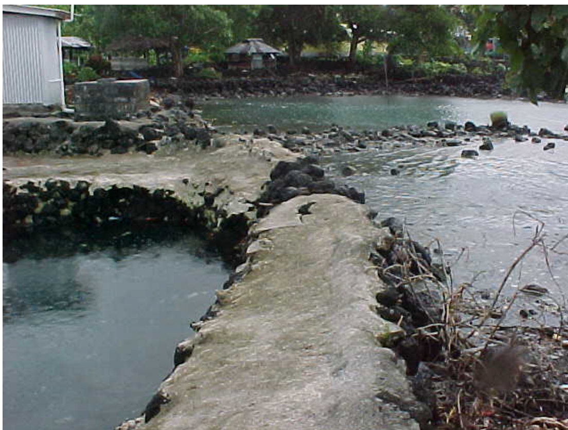
Vaitele Pool wall. Small rock construction and location results in high risk and susceptibility to damage.
