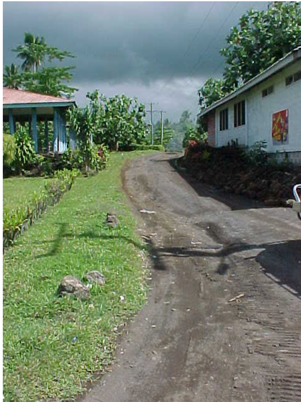
Work road intersection with Main Road showing scour along left hand side.
