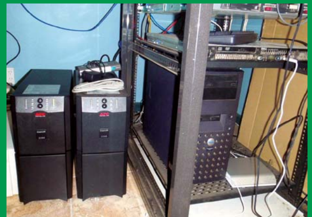
The current server in operation
